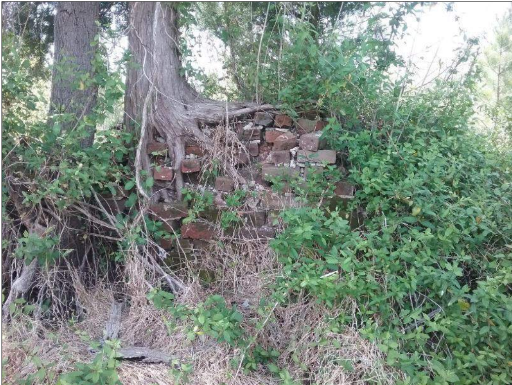
Figure 8-66: Cedar trees growing out of brick structure in Area E2, facing E.
