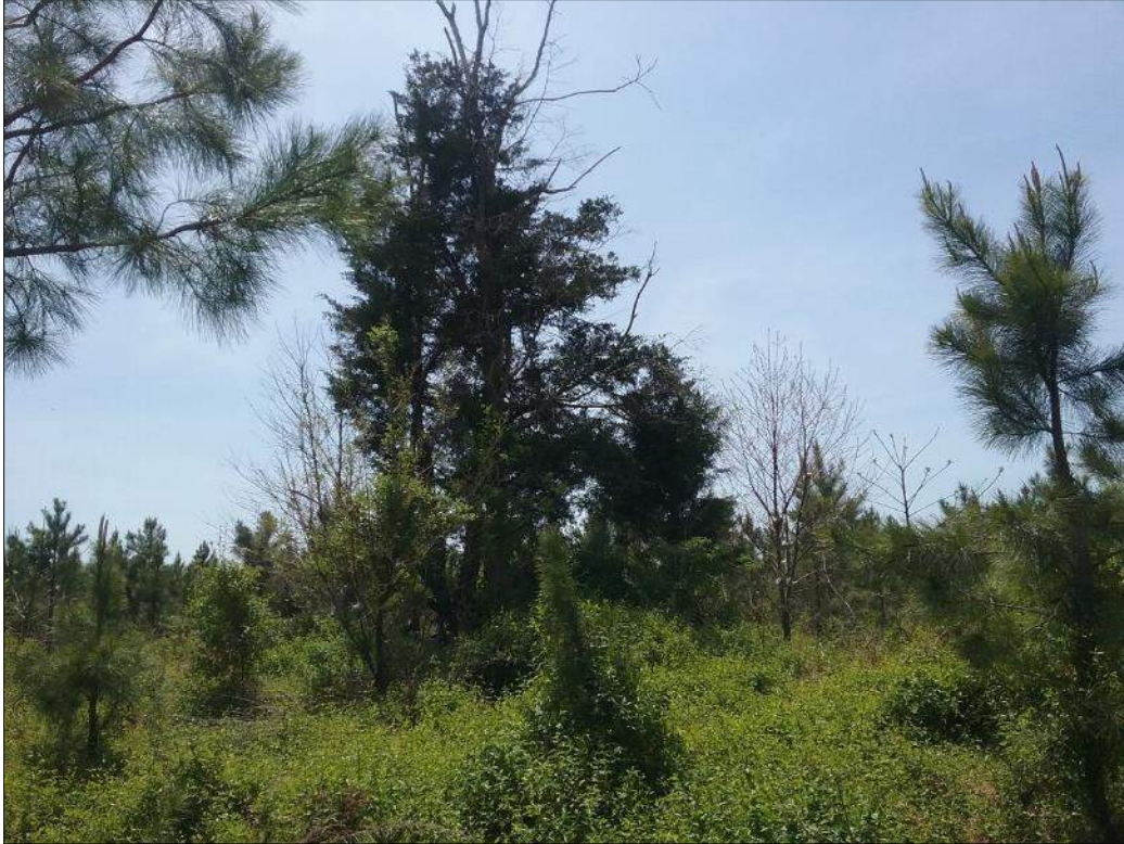
Figure 8-65: Overview of cedar trees growing out of a brick structure in Area E2, facing south.
