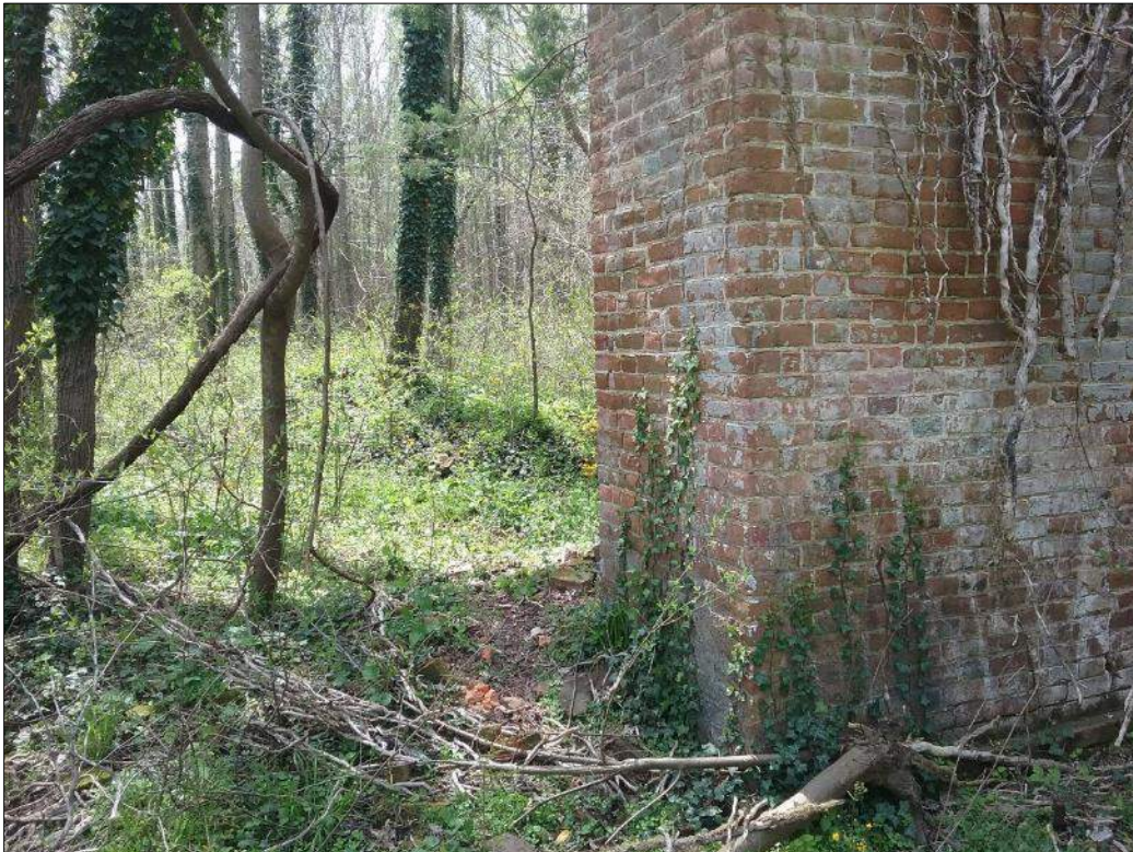
Figure 8-32: Chimney fall near standing chimney in Site 44LA0185.
